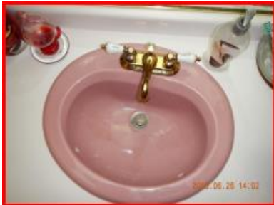
Basin and Drain Fixture:
