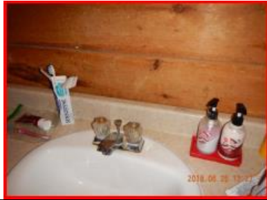
Basin and Drain Fixture:
