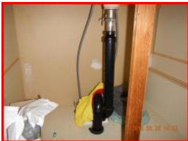
Faucet and Supply Lines: Toilet Condition
