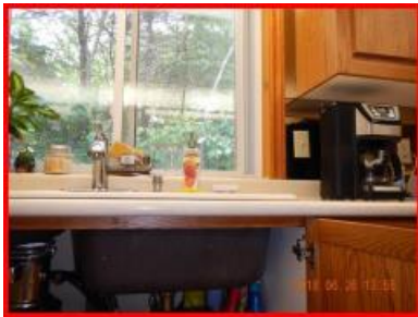
Sink and Drain Lines:
