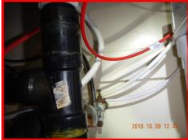
Sink and Drain Lines:
