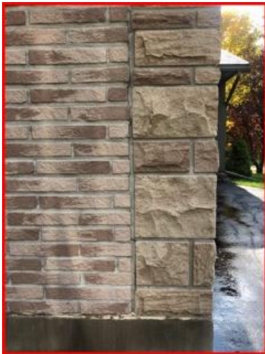
Evidence of Mould Noted:
