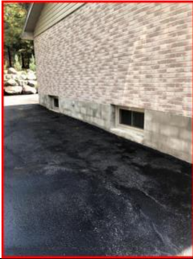
Earth-to-Wood Clearance: Structural Caulking:
